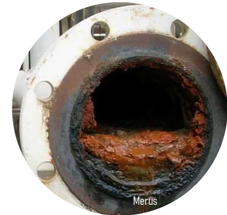
Biofouling in koelwatersysteem
